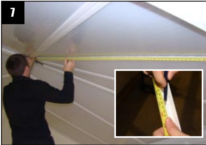
In a Victorian or splayed bar position, measure the length for the angle (same as the 'T' section). Mark the angle trim and cut to suit.
