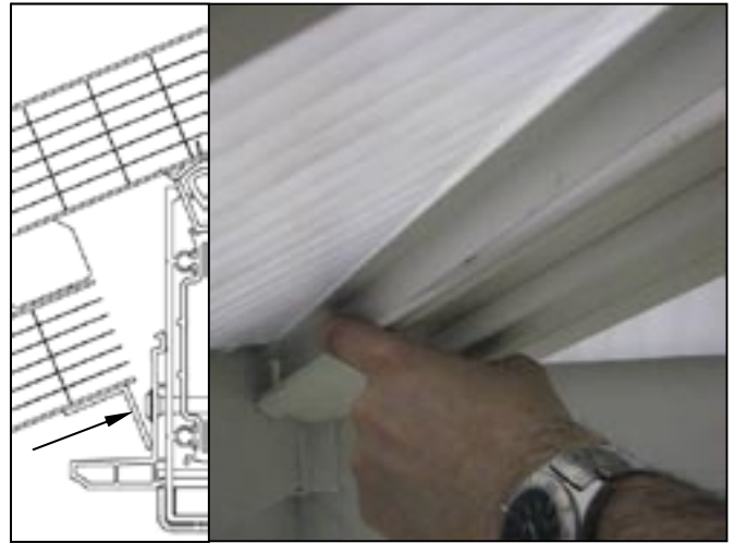
16. Cut BLAT001 or BLAX001 to the correct angle and length to run down the hip bar. Remove protective film off tape and apply to the underside of polycarbonate down the length of the bolster bar.
