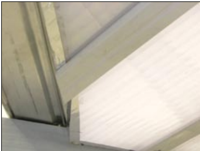
1. Fit internal layer of polycarbonate using the same process as for standard transoms.
