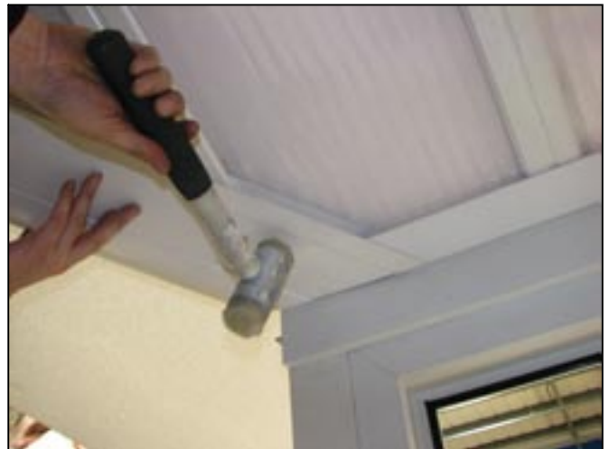
2. Fit valley undercladding as shown. Note: BLDC can be fitted before or after valley undercladding. (See step 6 for fitting after valley undercladding).
