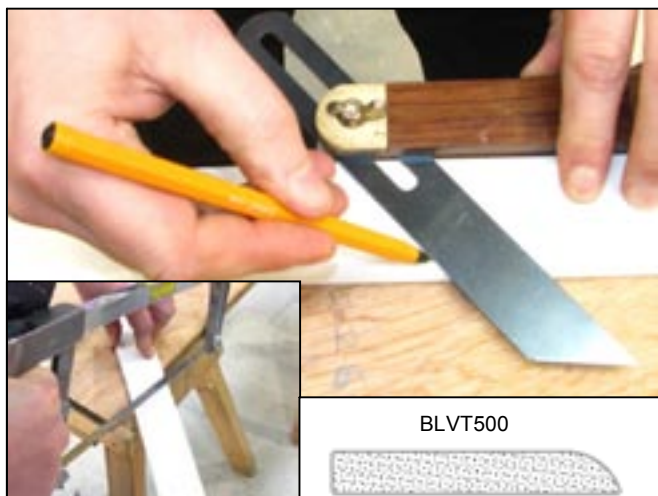
3. Measure the distance and angles between bars up the valley. Transfer measurements onto supplied architrave (BLVT500) and cut to suit.
