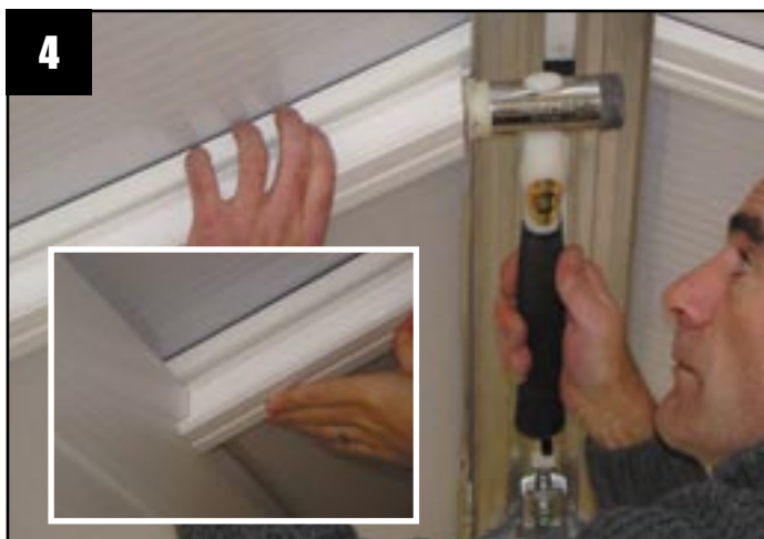
4 Lightly tap the 'T' section as shown for a tight fit against the fascia board.
