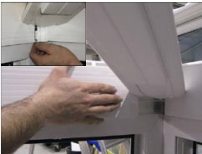
9. Slide opposite eaves fascia in behind hip bolster bar. Insert cut down corner between fascias and then continue to slide fascias until joint is tight.
