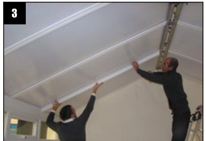
3 Offer up panel position 1 and the 'T' section and slide fit into the starter bar 'T' section. Clip fit into the glazing bar undercladding
