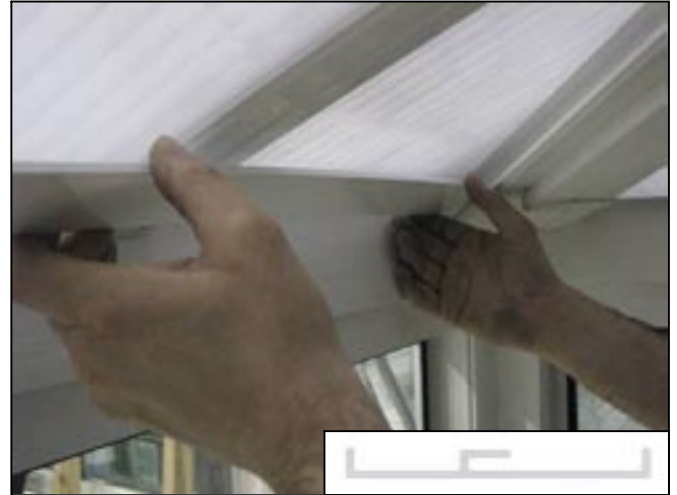
5. If fitting BLDC after valley cladding .Fit BLDC to brackets and tuck into hip L section.
