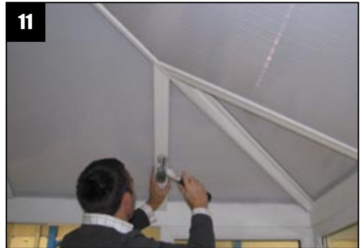
Fit the first jack rafter 'T' section to the glazing bar undercladding.
