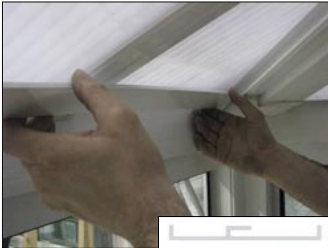
17. Fit BLDC to brackets and tuck into hip L section. In a valley situation tuck into valley undercladding.
