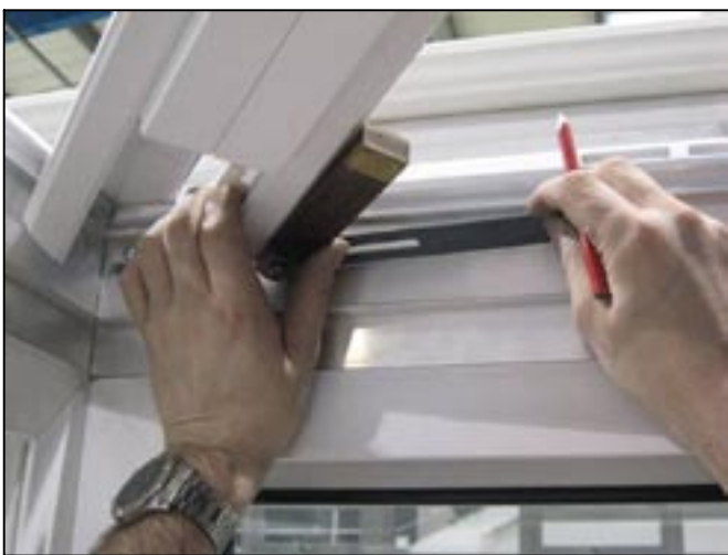
3. Using bevel or similar, measure angle of hip bar to the eaves as shown.
